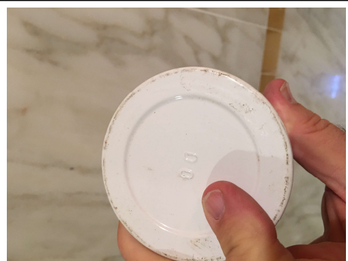
Bottom Year Mark on Kidde Fire Extinguisher
